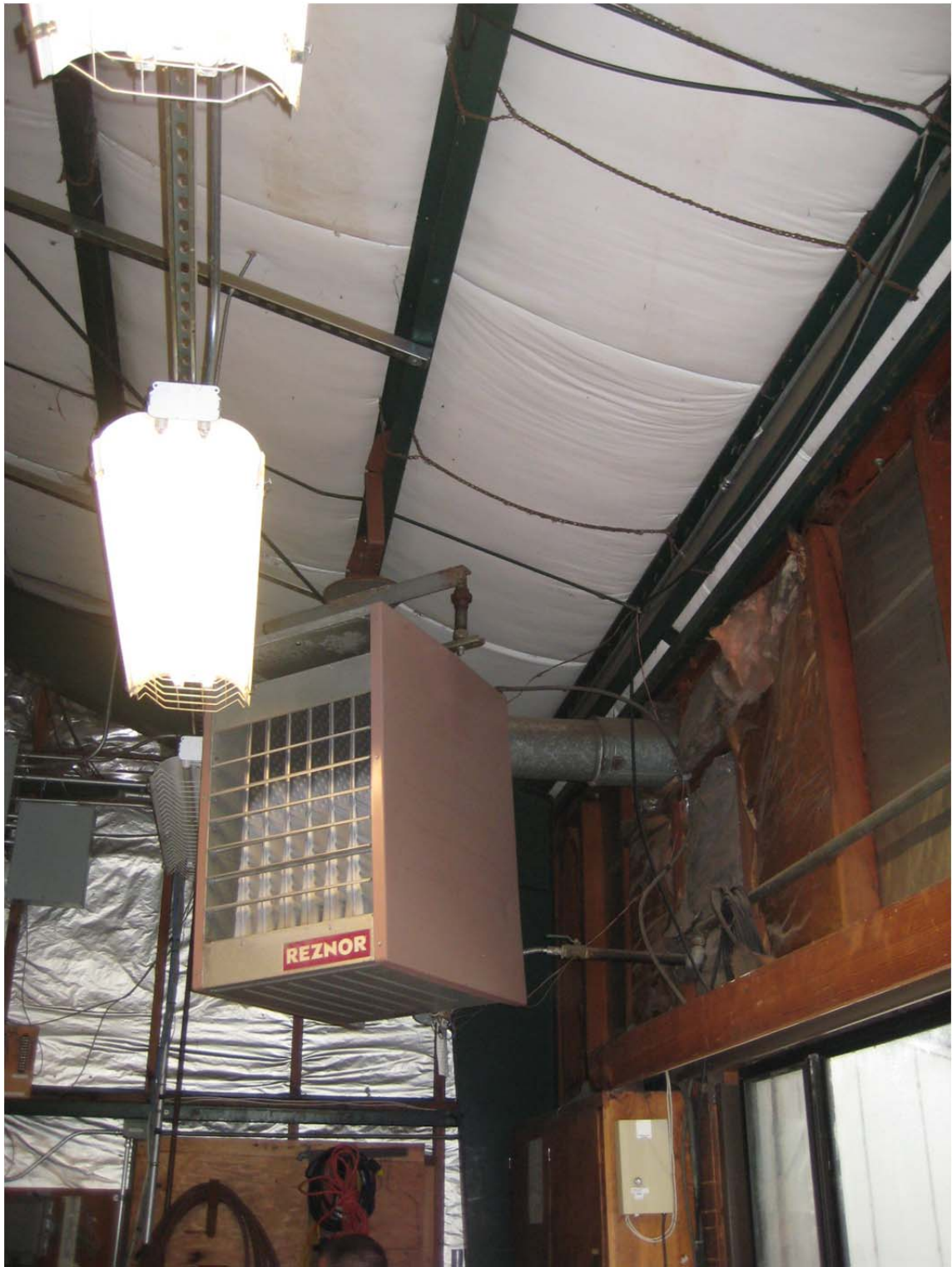
ME6 – Gas unit heater
