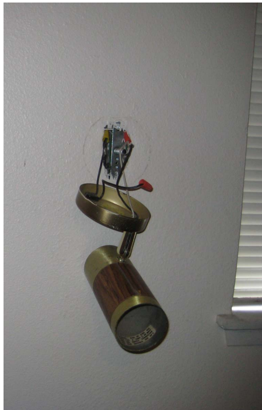
EE6 – Damaged light, Living Quarters
