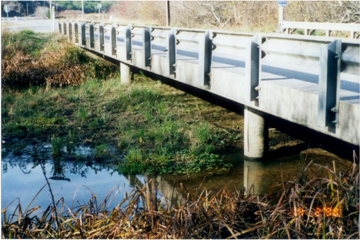
Pescadero Road Bridge Prior to Beaver Dam Removal (January 1999)
