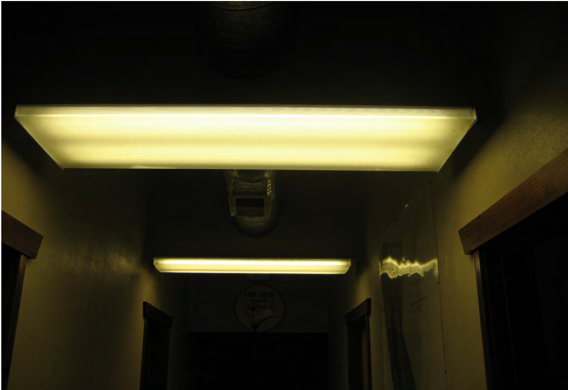
EE5 – Living quarters corridor lights
