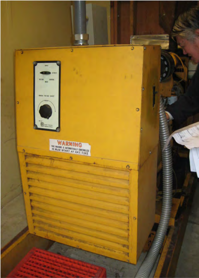
EE2 – Single phase diesel fuel standby generator
