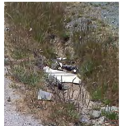
Storm drain lid (top); drainage culvert (middle); ponding area with collected trash (bottom)
