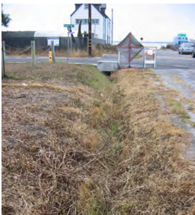
Denniston Creek mouth (top), shoreline exposed to coastal flooding (middle), and existing stormwater drainage ditch structures near Denniston Creek mouth (bottom)
