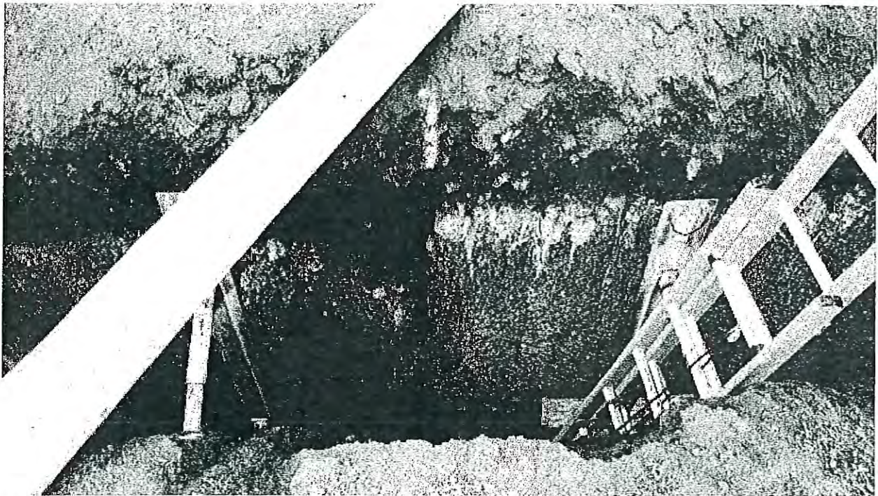
View of fault trace, north wall.
