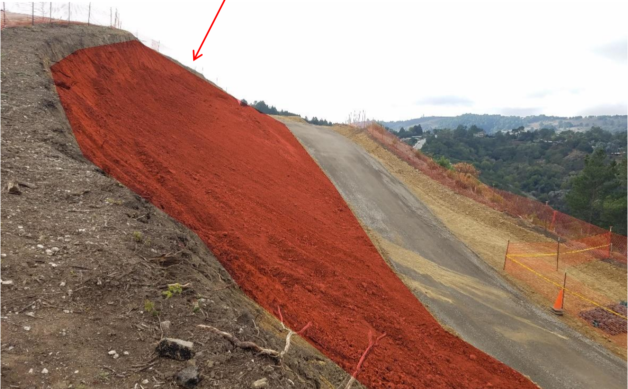
Figure 7: November 23 rd Erosion Inspection Mark-Up
