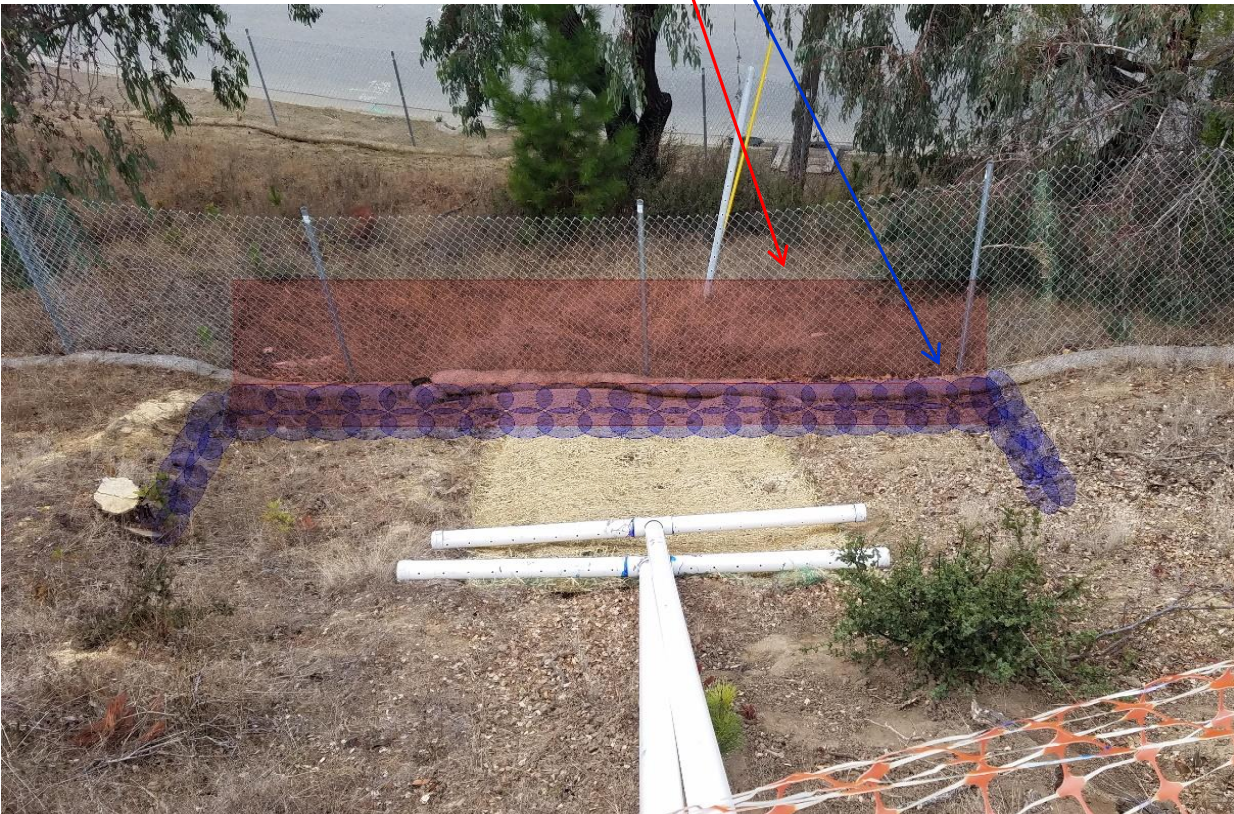
Figure 11: November 23 rd Erosion Inspection Mark-Up
