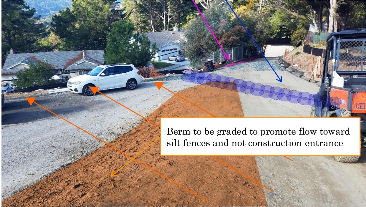
Figure 9: November 23 rd Erosion Inspection Mark-Up
