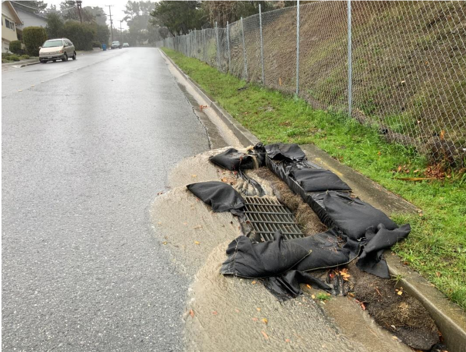
Figure 14: January 4 th discharge due to silt fence breach
